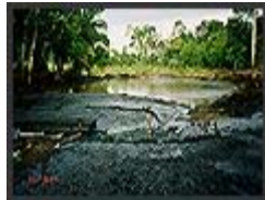
Land spill from pipeline
